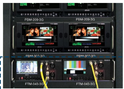
(2) FTM-043-3G units in Rack Mount - 2RU
